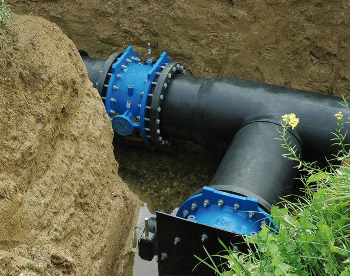
Figure 3.6. Installation with butterfly valves
