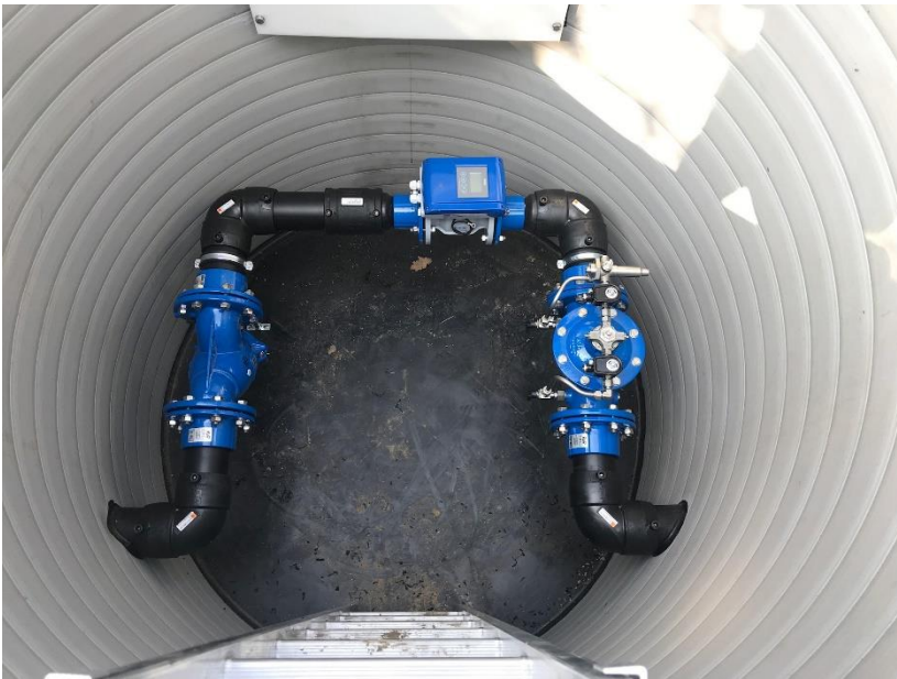
Figure 5.2. Control valve installation with new valves for pressure management
