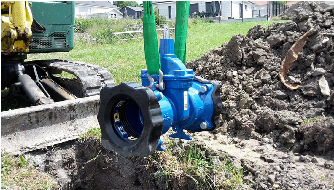
Figure 7.1. Operation and maintenance are very important to ensure a longer lifespan of installations and valves
