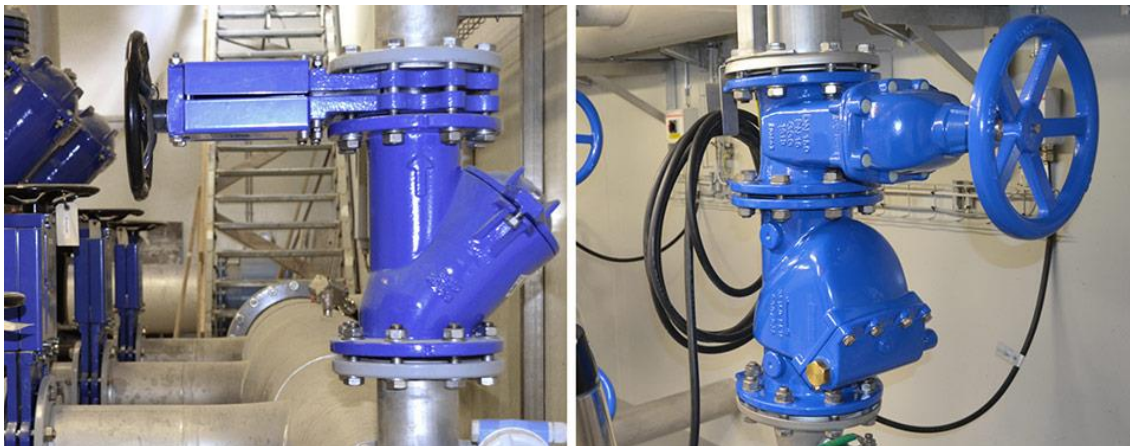
Figure 3.4. Installation with knife gate valve, ball check valve, swing check valve and gate valves
